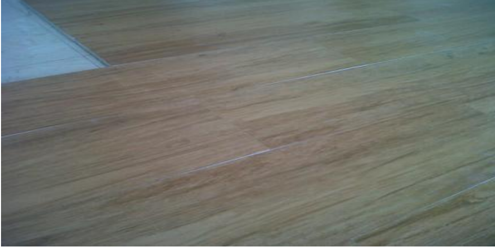
Brickway Laying %0 % Off set Wrong pattern shows warping at center
